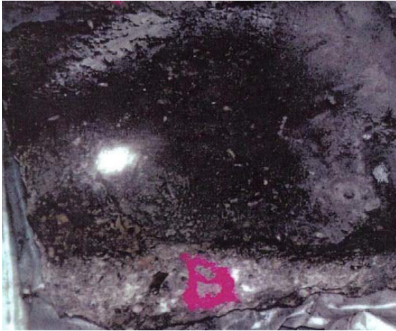
Top View Of Concrete Permeated With Oil
